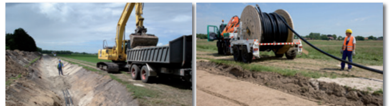
Along with the withstand test, the quality of the cable laying and installation is being increasingly combined with a PD diagnosis (pictures ABB)
